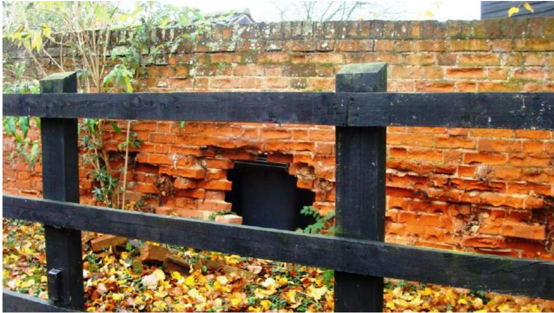
Picture 17. 19th century wall at Rennesley Farmhouse in urgent need of repair. The potential of grant assistance from EHDC exists.
