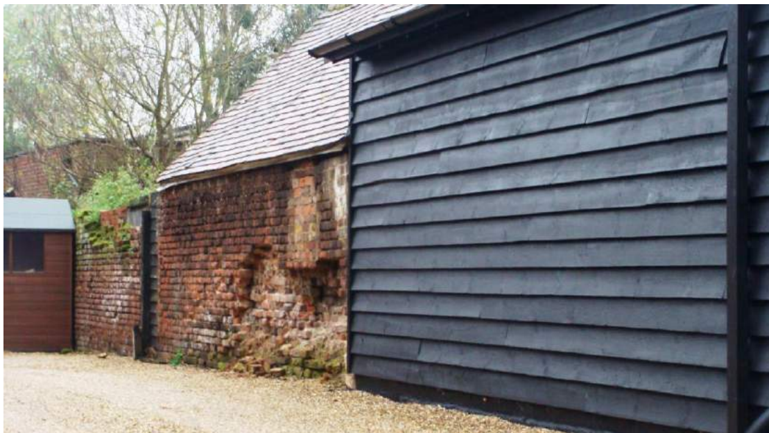
Picture 15. Ancillary building assumed to form part of Trinity Barn complex whose brickwork is in need of repair.
