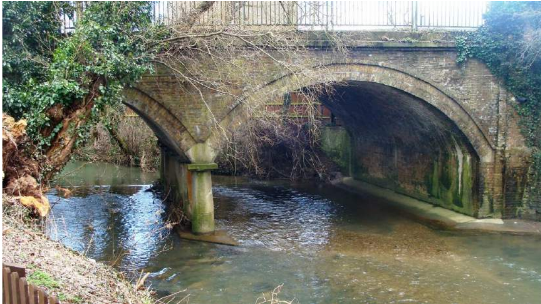
Picture 5. Listed road bridge over River Rib. Considered to be very fine in some of its detailing.
